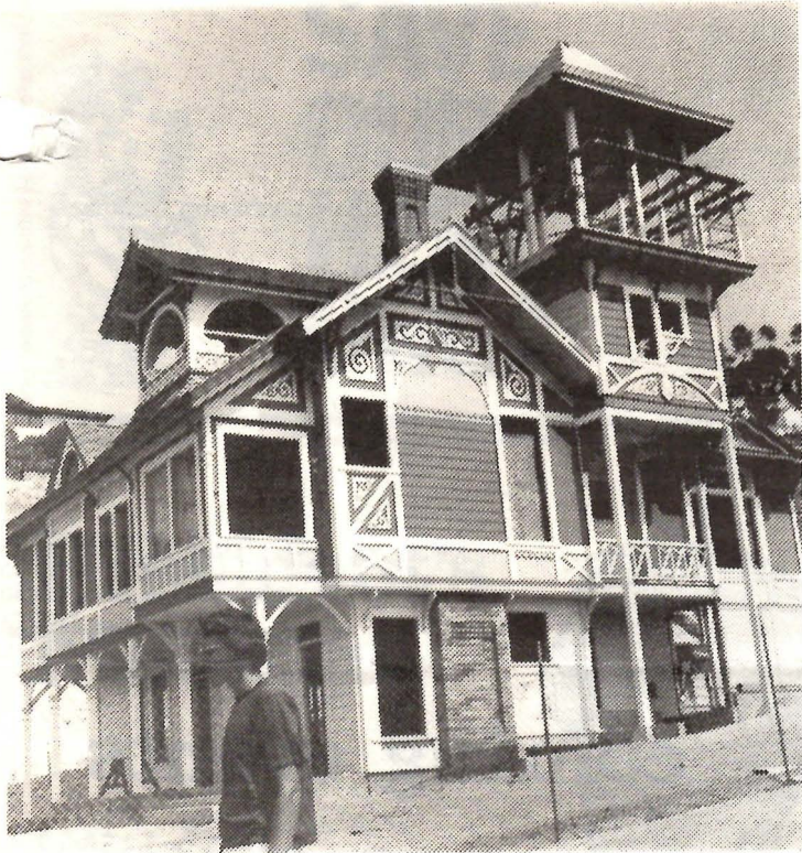
THE SHERMAN-GILBERT HOUSE—A VIEW OF THE PROGRESS BEING MADE AT HERITAGE PARK IN OLD TOWN. THIS PHOTOGRAPH WAS TAKEN ON SEPTEMBER 28TH OF THIS YEAR. THE TOWER IS NOW COMPLETED. WORK BEGAN ON MOVING THE SHERMAN-GILBERT HOUSE IN MAY, 1971.
