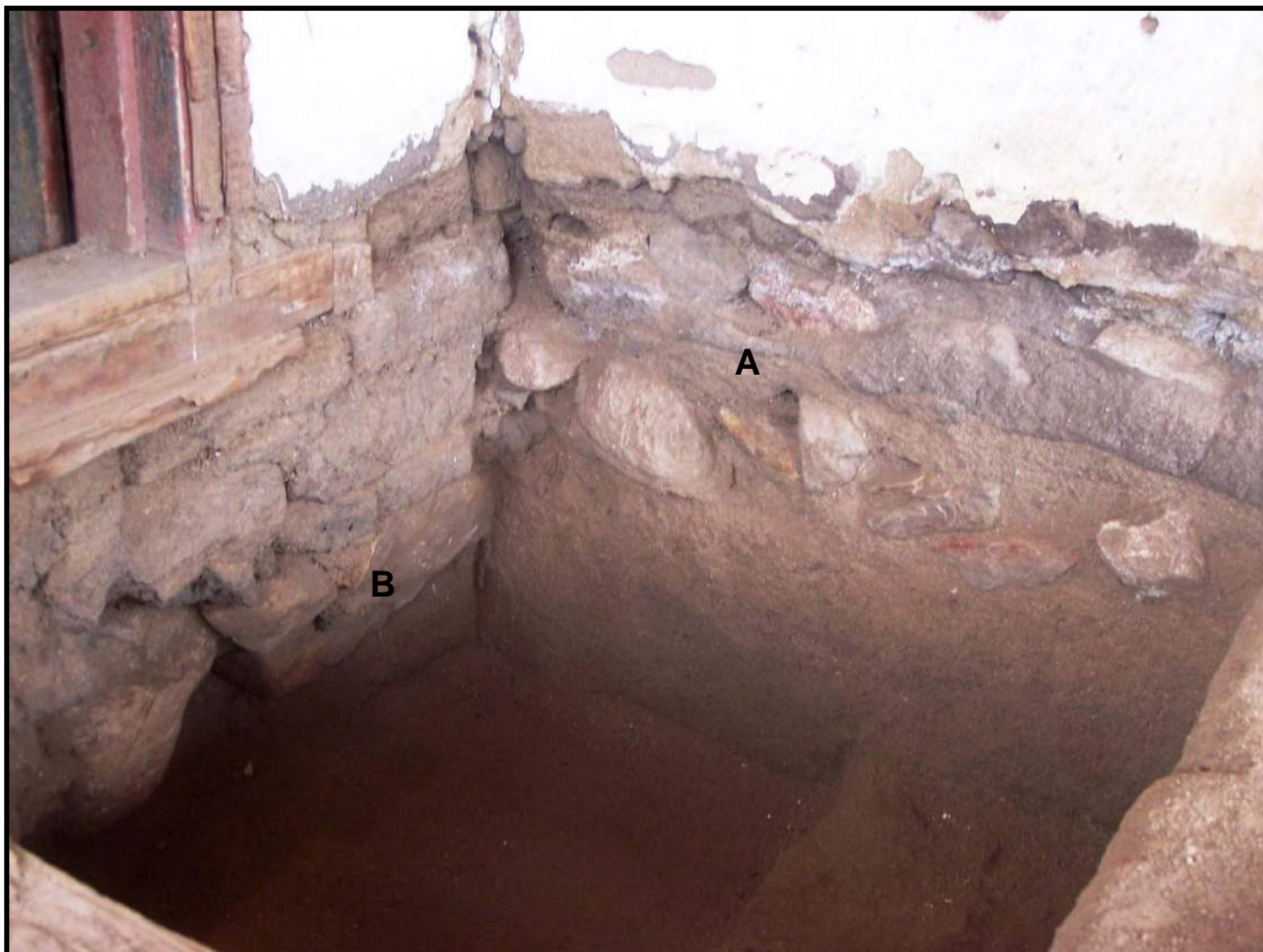
Figure 59: Unit 3, Room 104, showing the west wall foundation of Room 103 (A) and the relationship between the angular granite field stone footing of the Central Wing (B).
