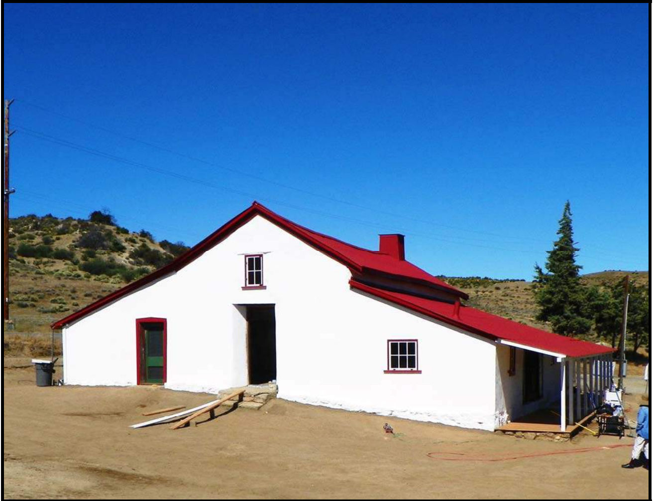
Figure 19: In July 2011, restoration work was completed along the east side of the Ranch House.
