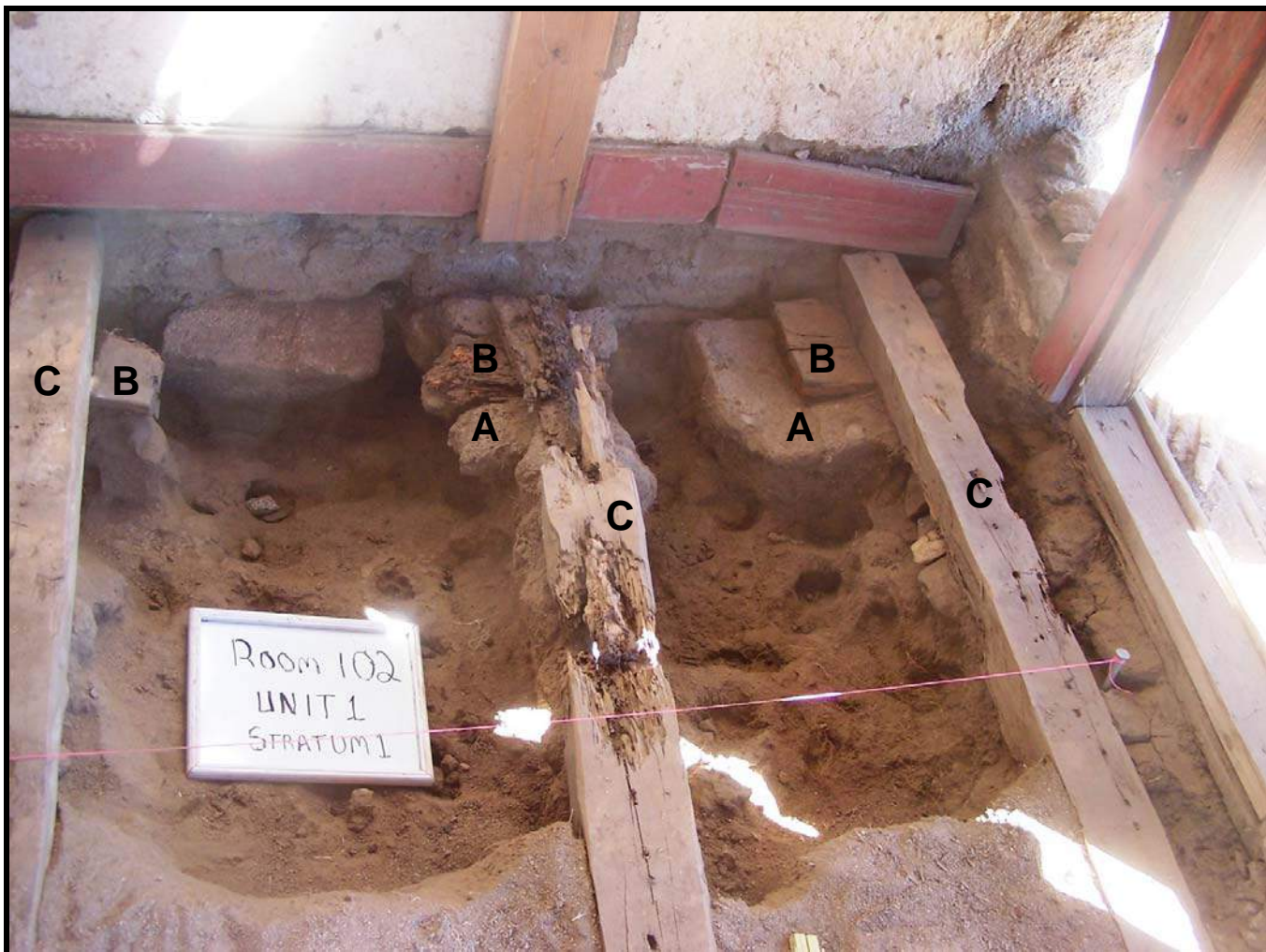
Figure 61: Unit 10-1 excavated to 12 inches below surface. Note the large number of rodent burrows and the adobe blocks (A) supporting wooden boards (B), set under the floor sleepers (C).
