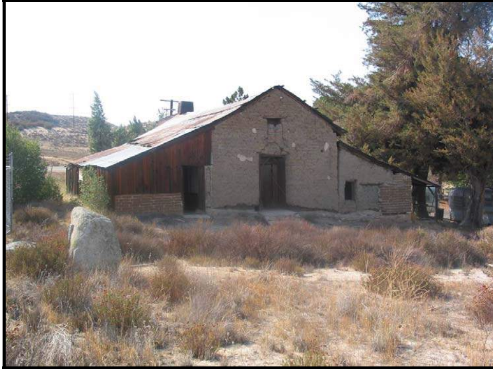
Figure 26: The east façade vividly illustrates the three different sections of the structure. The original two-room adobe can be seen in the center with the adobe addition to the north (right) and the wood/adobe addition to the south (left).
