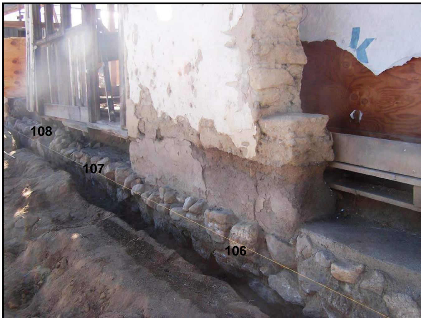
Figure 76: North wall foundation of the North Wing exposed in the restoration construction trench along the northern edges of Rooms 106, 107 and 108. The segment at lower right was capped with concrete during stabilization activities in 2004.
