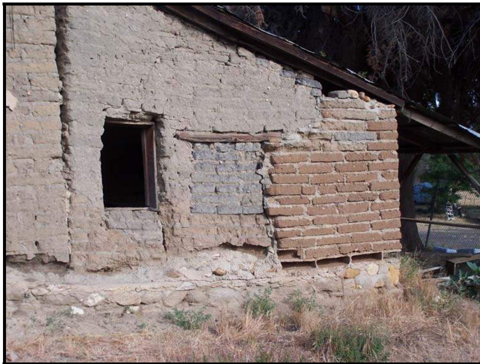
Figure 27: Multiple phases of construction can be seen in the east wall of the North Wing. Note how the wall is pulling away from the Central Wing on the left, suggesting a later period of construction.
