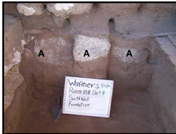
Figure 28: Angular granite fieldstones in the north wall footing of Room 101 (A), as seen in the south wall of Unit 10-4 Room 108. These are typical of the angular granite stone used throughout most of the foundation of the Central Wing.
