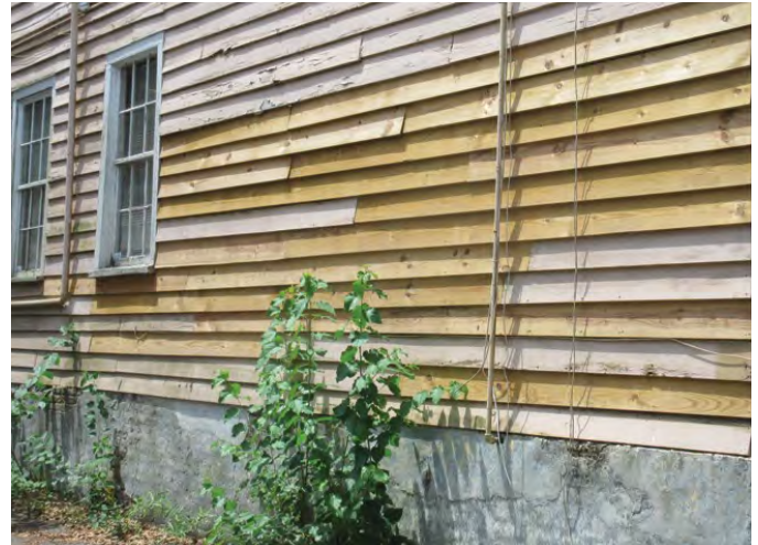
Figure 3: Incremental repair is best done using in-kind material to minimize differences in the performance characteristics that could negatively affect the overall assembly. Photo: NPS.
