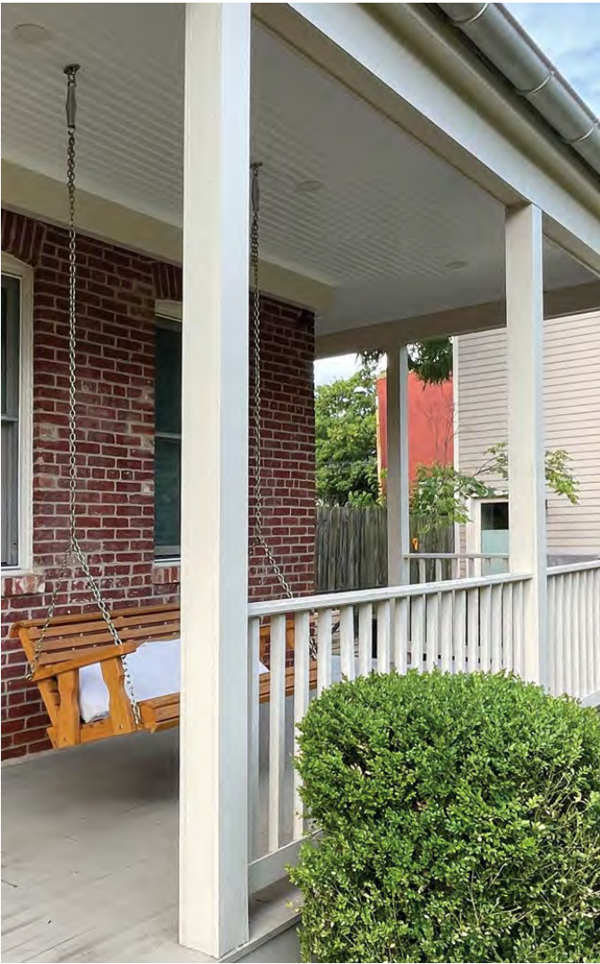
Figure 22. A porch was reconstructed using posts fabricated on site from a smooth-surface cellulose/polymer composite material. Though the face of the posts are painted, the lack of paint on the bottom at the cut ends is not consistent with manufacturers' recommendations. This treatment will allow moisture to be absorbed, shortening the life of the new replacement feature. Photo: John Sandor, NPS.
