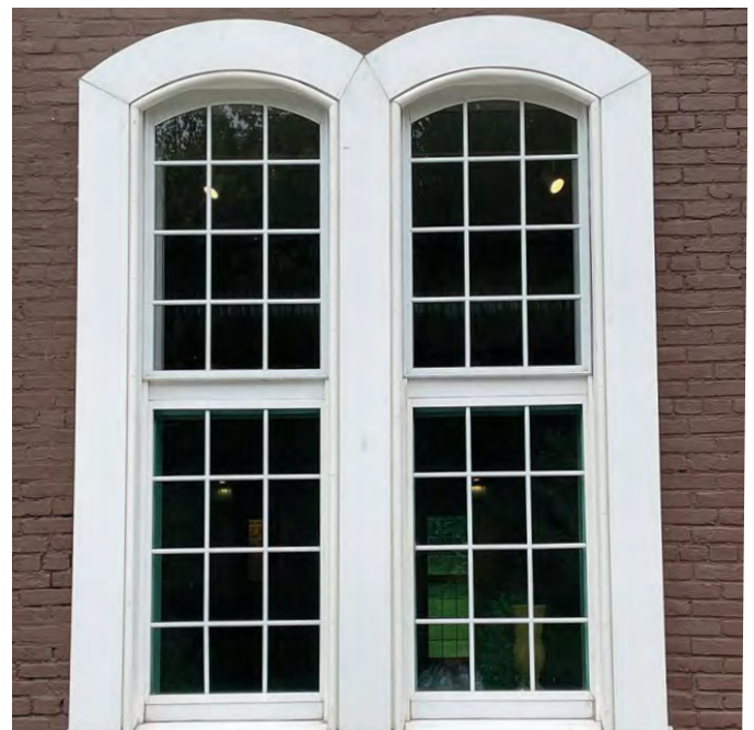
Figure 9. Previously bricked-in openings below the flood line were reopened and new aluminum windows installed with cellular PVC trim detailed to hold back moderate flood waters and survive exposure to water. Photo: John Sandor, NPS.
