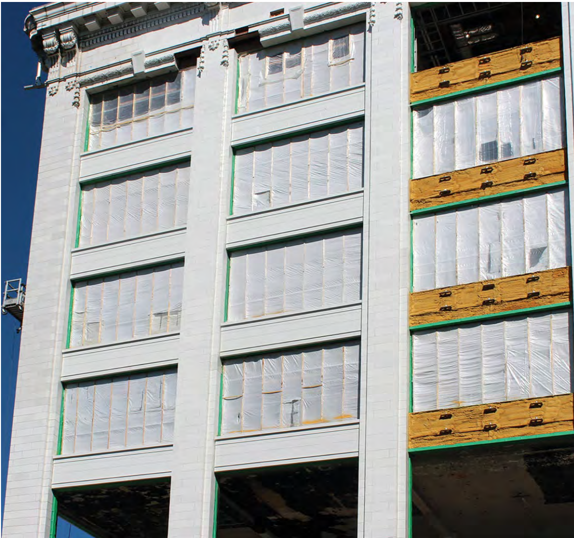
Figure 18. Missing historic terra cotta spandrel panels on all floor levels were recreated utilizing glass fiber reinforced concrete (GFRC) replacements. New spandrels were fabricated as individual components and attached with metal terra cotta piers. Photo: Kris Frail, Dewberry.
