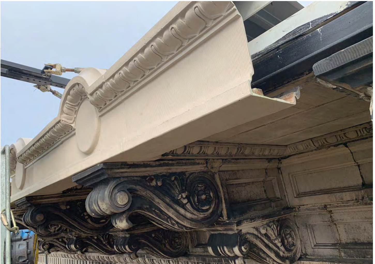
Figure 19. A new, lightweight fiber reinforced polymer is attached to a new metal armature to replicate damaged and missing elements of a terra cotta cornice. Photo: Quinn Evans.
