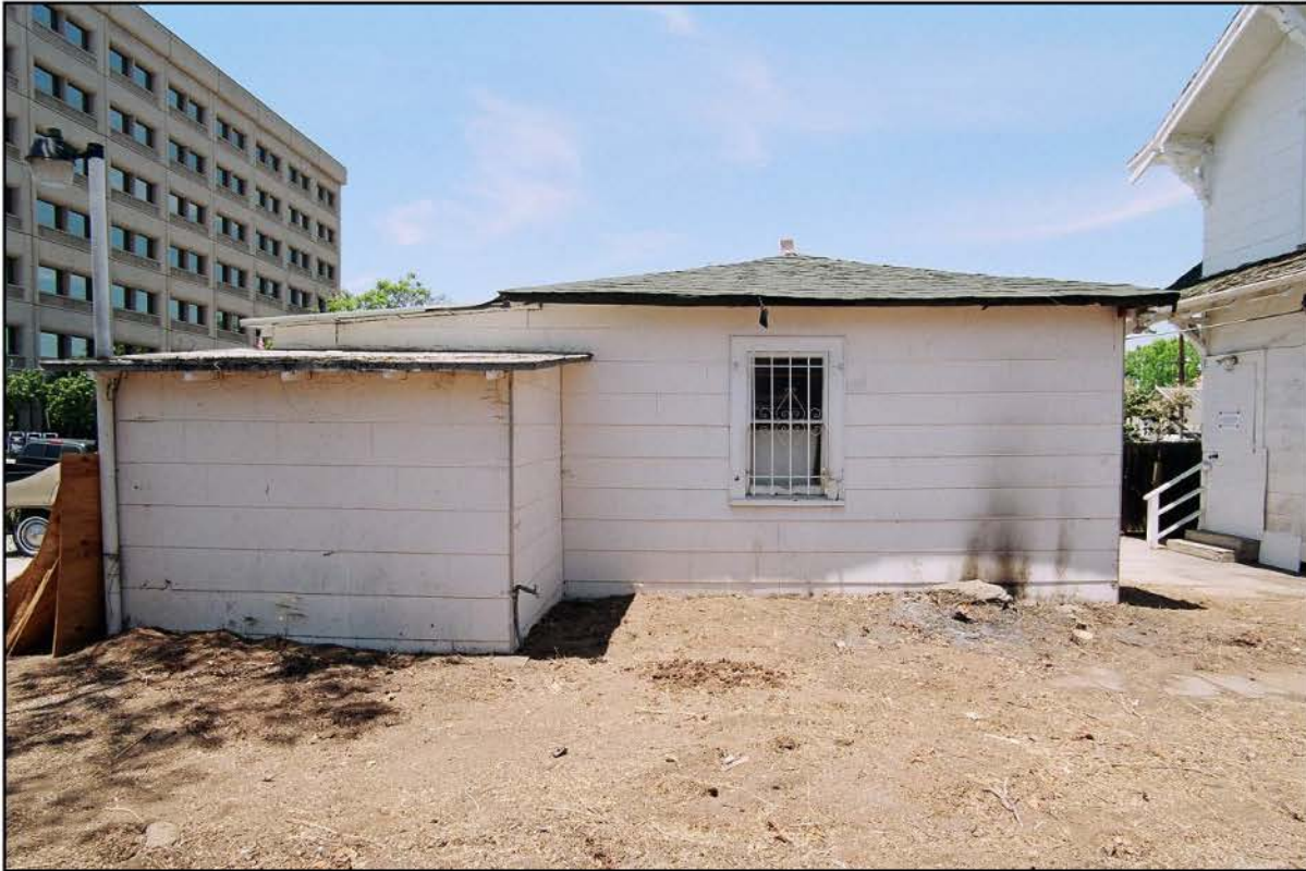
Photograph 30 Overview of Garage Building, Taken Before Siding Was Removed, Showing Relationship of Addition (on Left) to Original Garage
