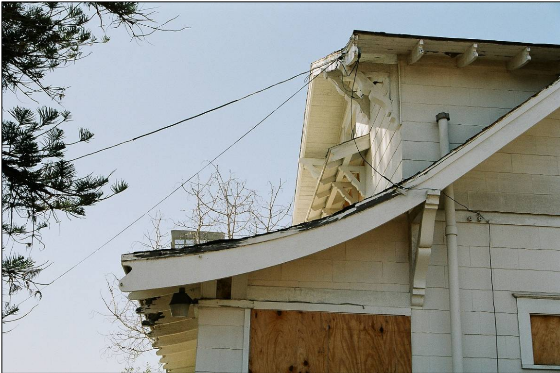
Photograph 3 Main Roof and Dormer Roof Eaves, Showing Rafter Curve and Decorative End Cuts
