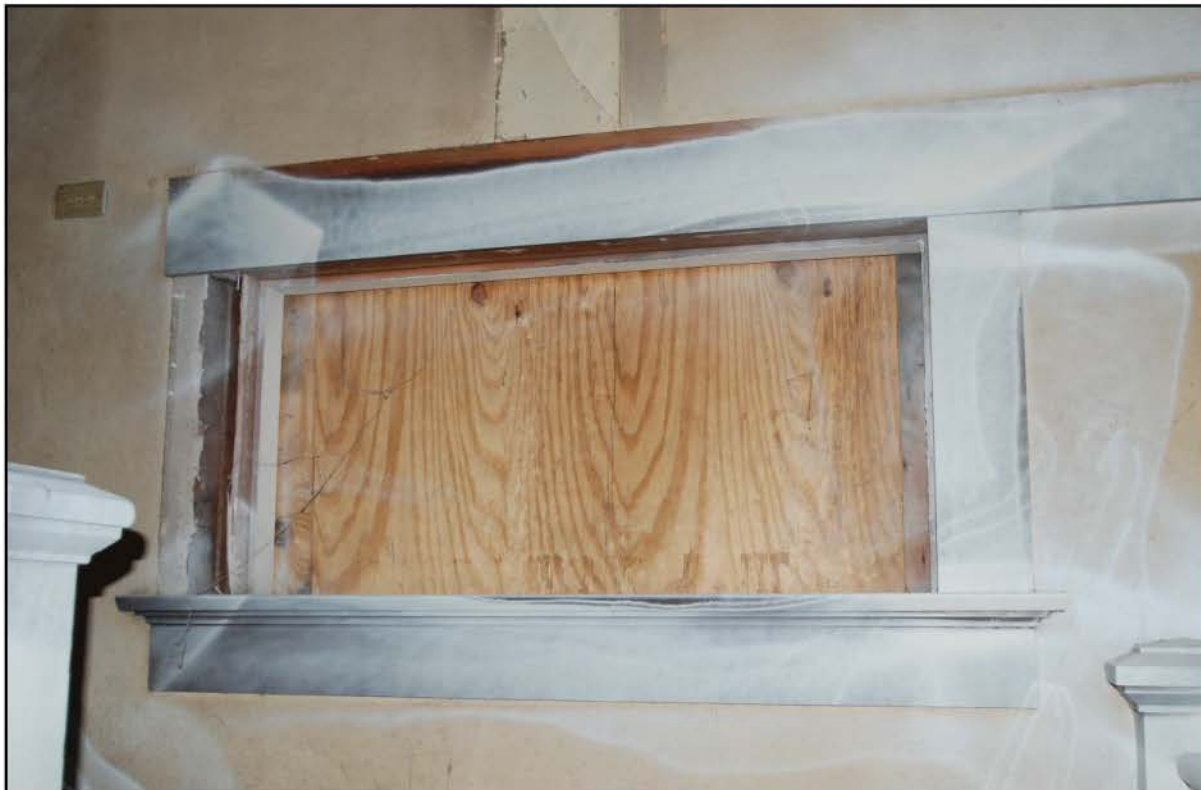
Photograph 15 North Side Window 2, Interior Shot, Showing Missing Sash
