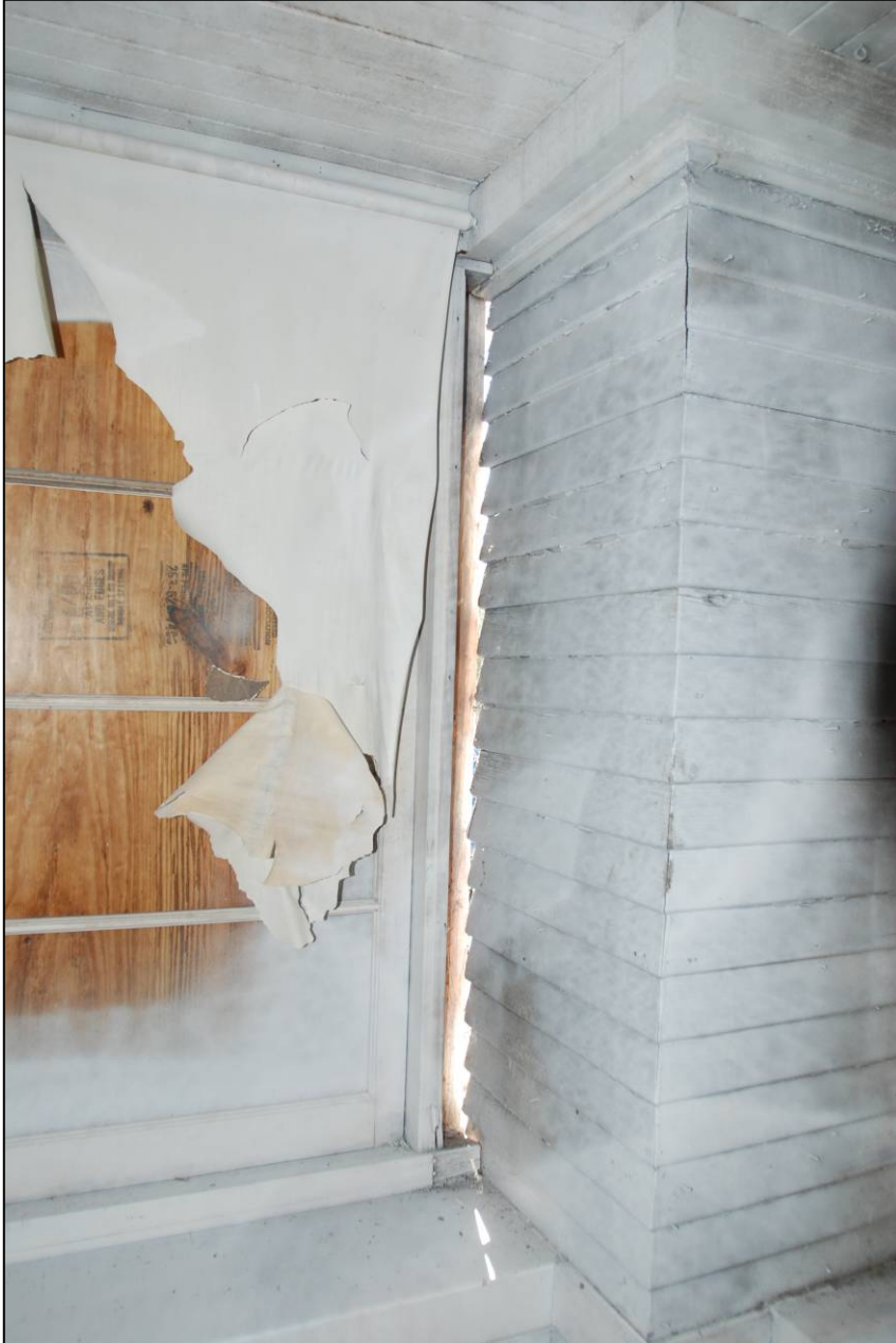
Photograph 11 Interior View of Porch Window Showing gap Between Window Frame and Porch Clapboard
