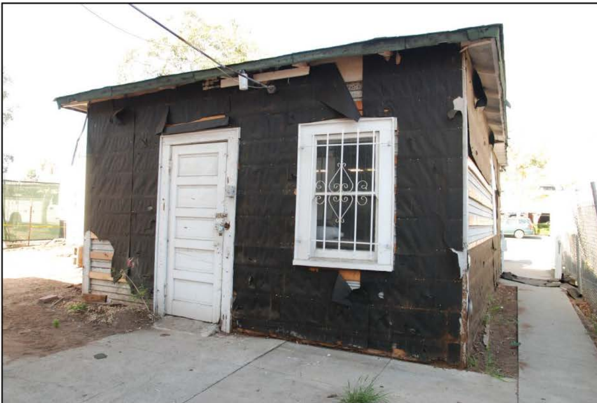
Photograph 29 East Side of Garage, Current Condition. Note Different Style of Window Casing
