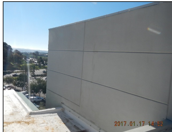
Figure 12: Antennas are concealed within the left-hand side of this wall.
