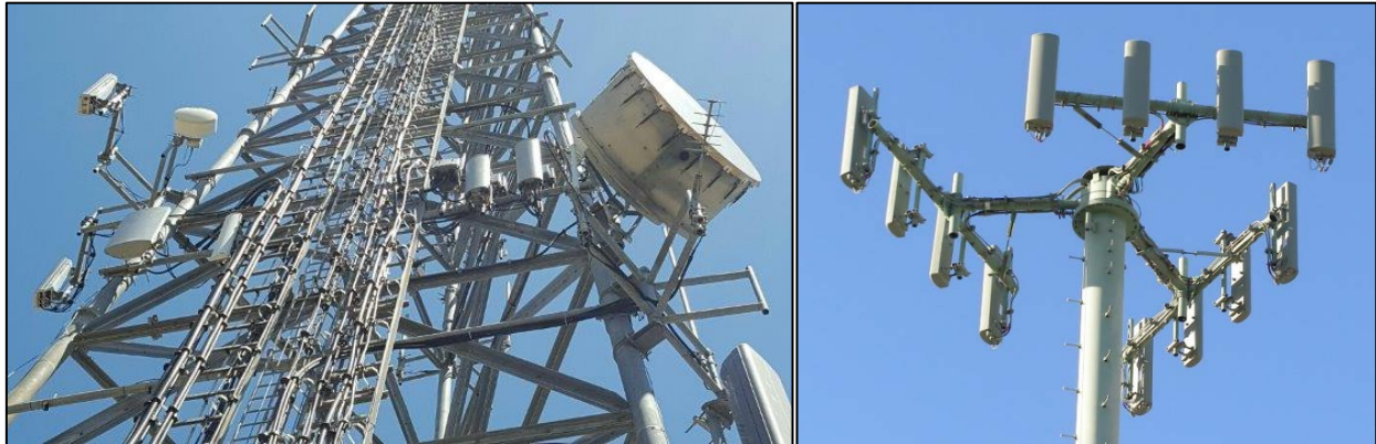
Figure 33: Lattice towers and monopoles don't integrate. They do not meet the requirements of the Wireless Ordinance.
