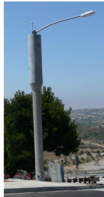
Figure 26: Macro (non-small cell) right-of-way site with antenna shroud
