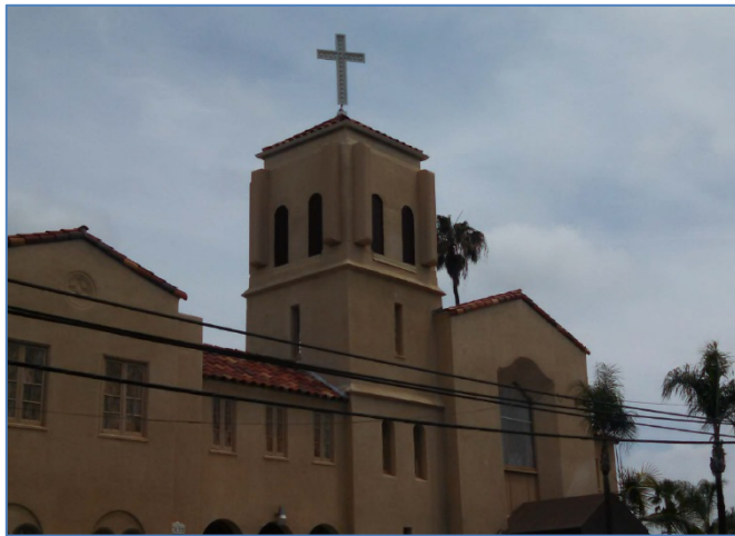
Figure 14: Façade-mounted antennas with antenna skirts and chin straps, placed symmetrically and painted to match.
