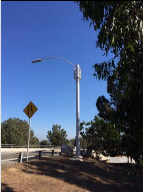
Figure 27: This right-of-way installation has three antennas mounted flush to the pole with no pipe mounts and no antenna shroud. This is an older installation with no chin covers; they are now required.
