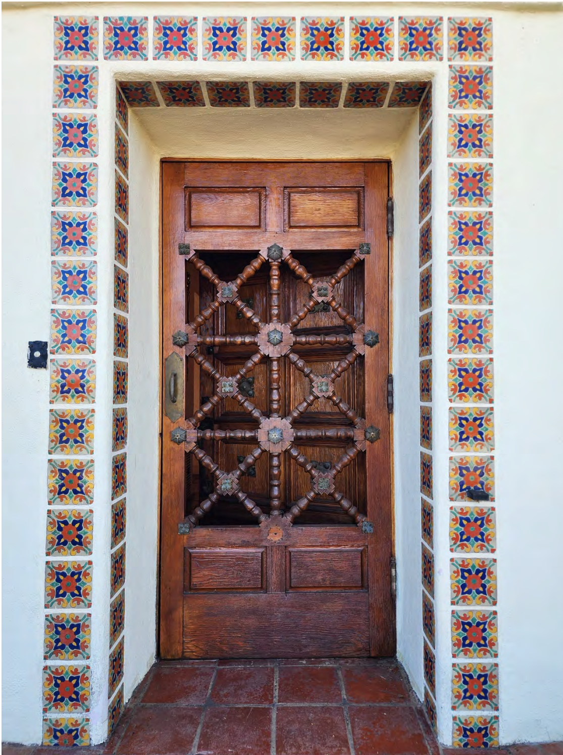
Photo 5a: The main entryway is set within a recessed opening, framed by decorative hand-painted tiles. The wood entry door, original to the dwelling, is highly detailed, featuring a geometric spindle work and ornamental metal accents. Source: Urbana Preservation & Planning, LLC.
