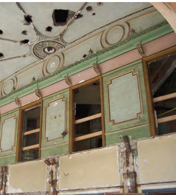
Below A flat 1950's ceiling was removed from the entry rotunda, revealing that much of the plaster ornamentation was missing or damaged, the upper floor windows were gone, and there were gaping holes in the walls and vaulted ceiling. The pink and green colors were also not historic.
